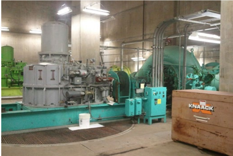
Fig 1: John Day South Fish Turbine Pump #2
